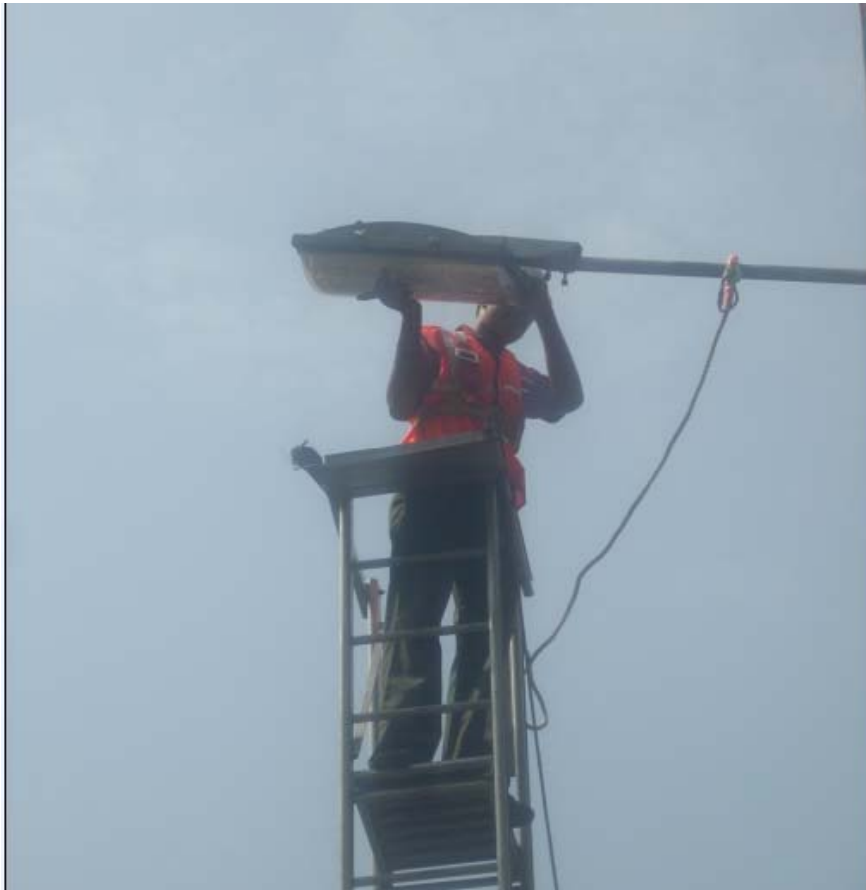
SAFETY BELT USED HOOKED ON THE LADDER AND THE POLE BRACKET DURING INSTALLATION AND MAINTENANCE
